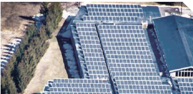
Super Market, Canada - SPV Capacity: 800 kWp
